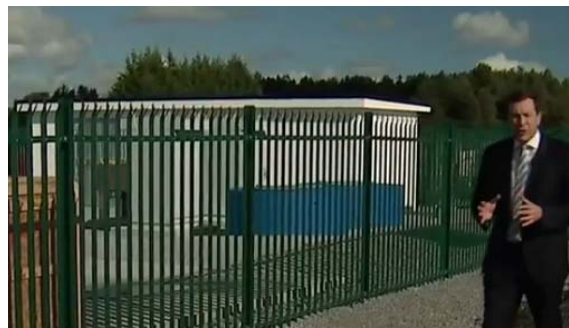
Figure 11 - Two modular Beacon FES systems installed in Ireland for Schwungrad Energy as a renewable / battery hybrid demonstration.
