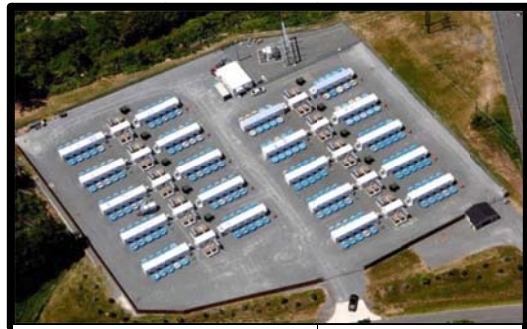
Figure 9 - Beacon FES Stephentown, NY, 20 MW, Operating since Q1 2011
